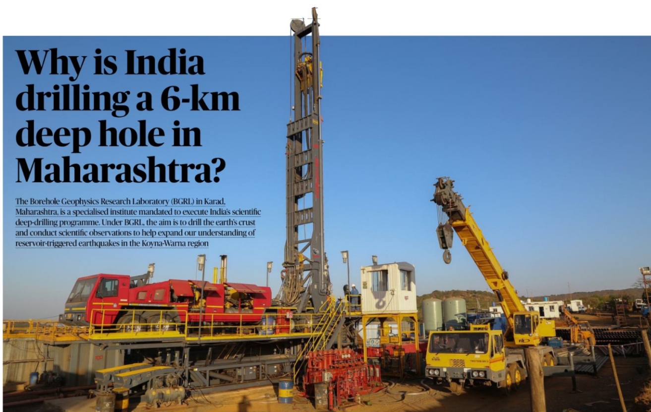
DEEP DIVE: At the deep drilling site in Koyna region, Maharashtra, the towering drilling rig is seen surrounded by associated equipment, an onsite mud logging unit, gas analysis lab, and a geological studies lab. MOES-BGRL
